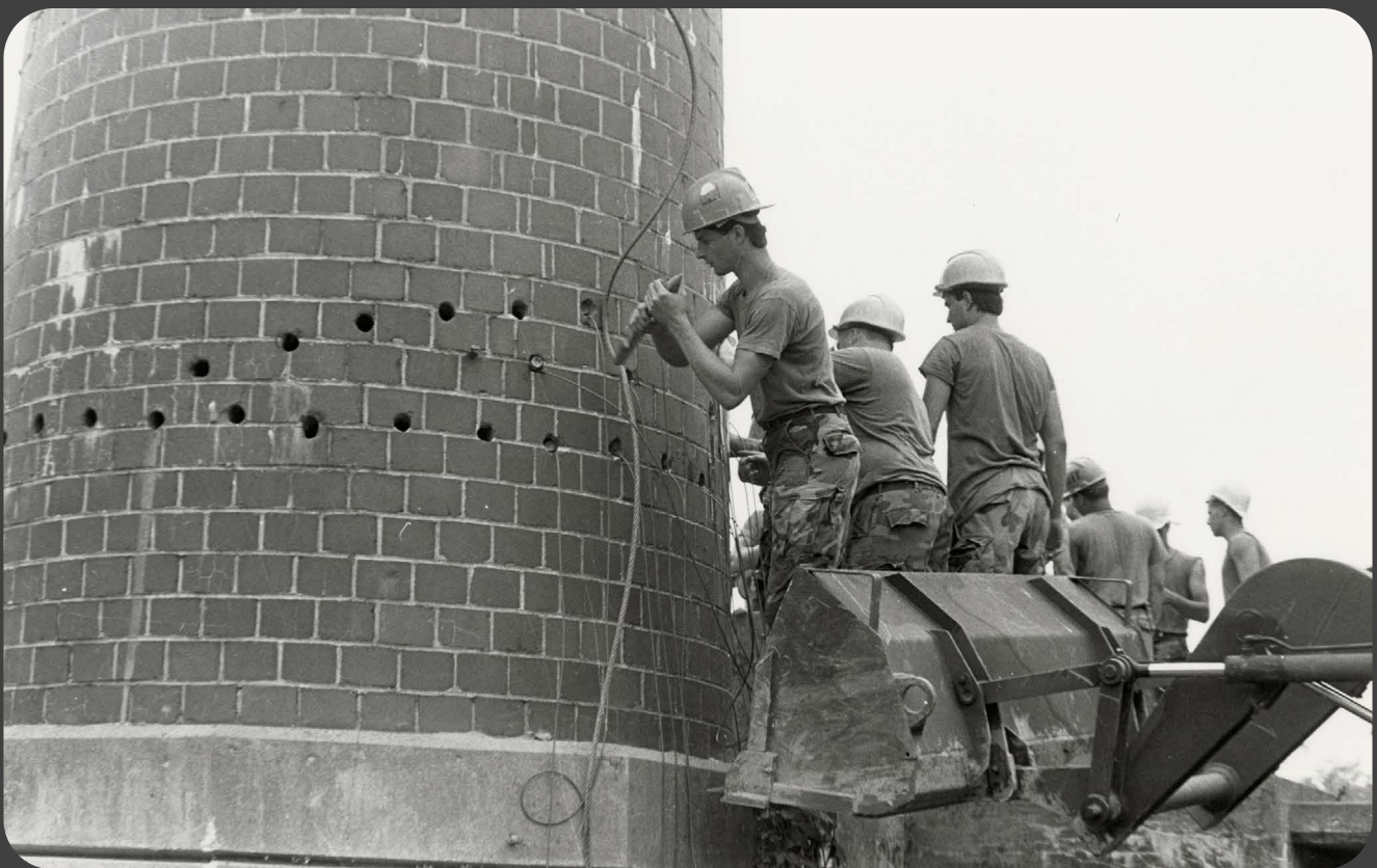
Soldiers from Company C, 112th Engineer Battalion place explosives charges on the outside of a chimney at Camp Atterbury, Ind., on June 21, 1991, prior to demolishing the structure.
